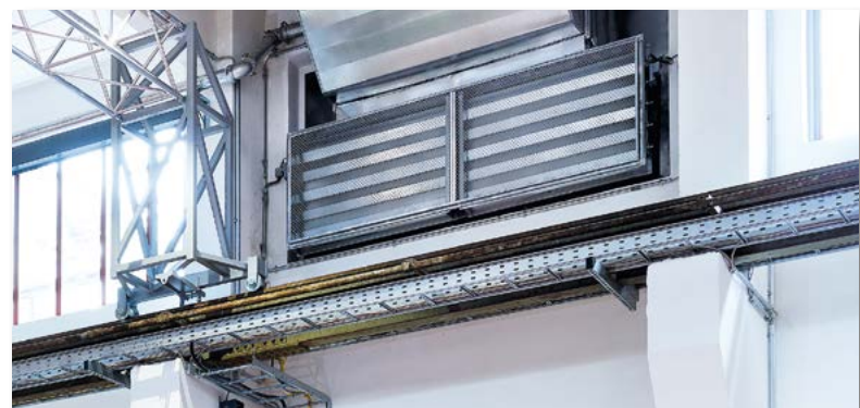
In the event of a fire, air is supplied by means of noise-insulated multileaf dampers, special supply air inlets and the main stairwell. An air handling unit also supplies a considerable portion of the additional supply air.
