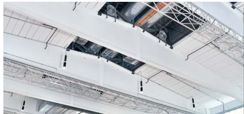
Ten BVAXN smoke exhaust fans remove the smoke in the event of a fire.
