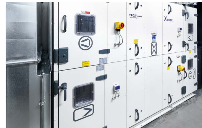
A small X-CUBE air handling unit in the basement removes the extract air from the catering area if required.
