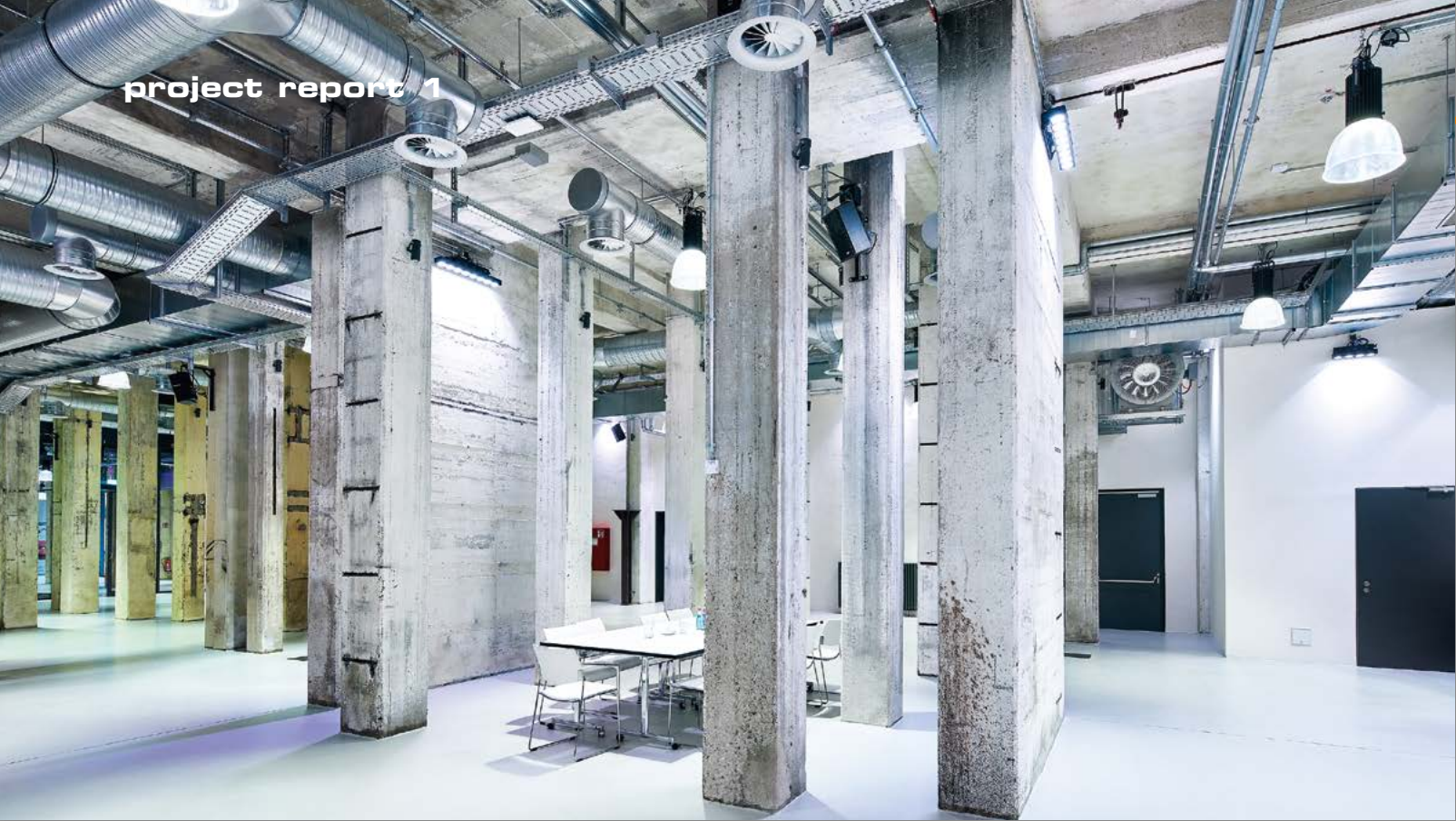
Ducts and swirl diffusers are installed exposed to add to the industrial style of the ground floor lounge and bar area.
